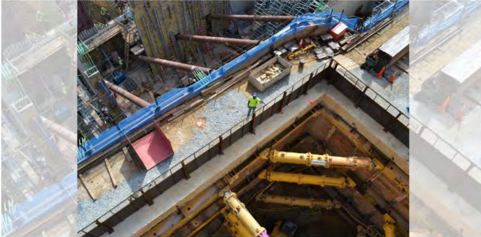
Construction work on the Bethesda shaft of the Maryland Purple Line Light Rail project. Photo courtesy of the Maryland Dept. of Transportation
